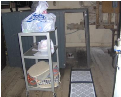
The door with its air filters for the cabinet housing the Spencer Blower was on the floor.
